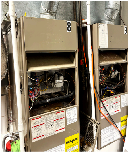
Existing 40-year-old HVAC units in north wing.
